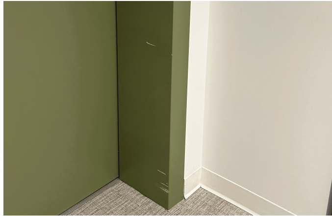
Figure 3: Dents and wall damage caused by wheelchair crashes
